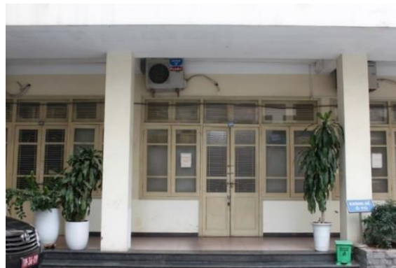
Figure 3: Adding ductless mini-split system air conditioner to offices at the Ministry of Education Headquarters
